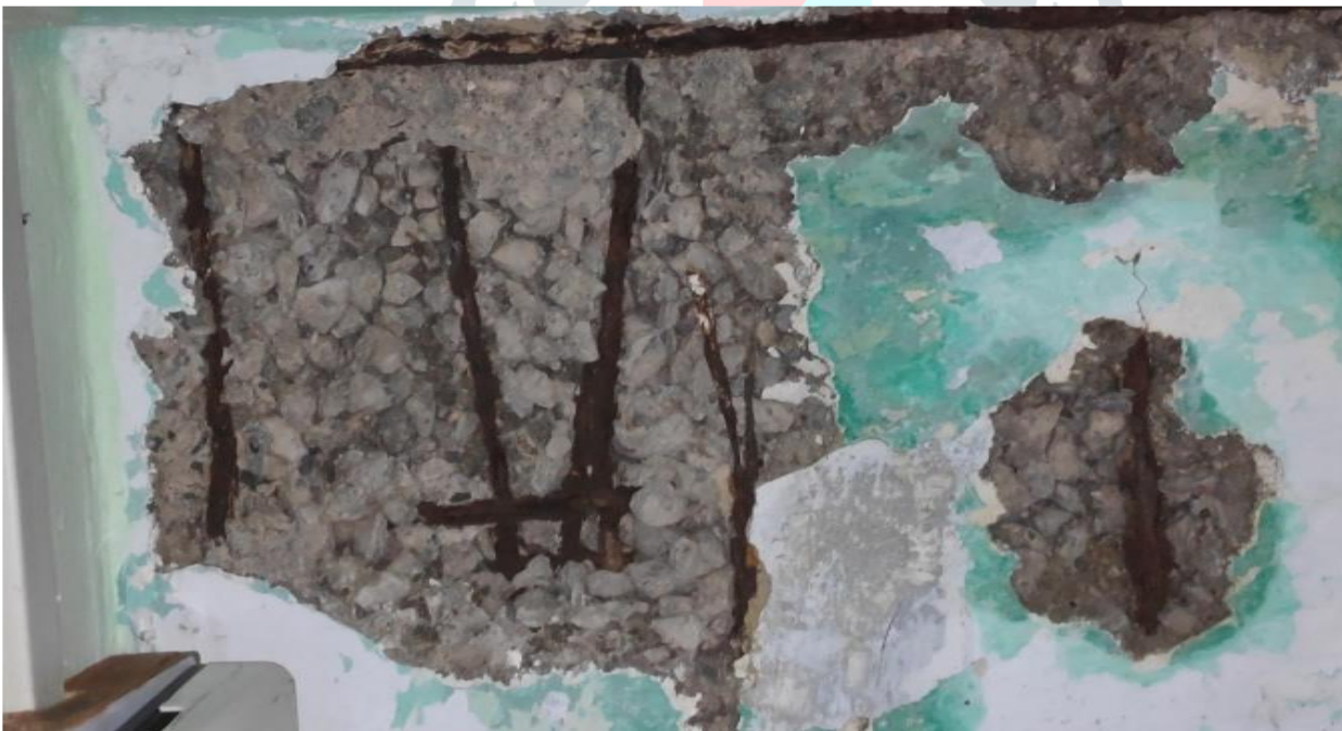
Fig.1– Totally damaged slab
