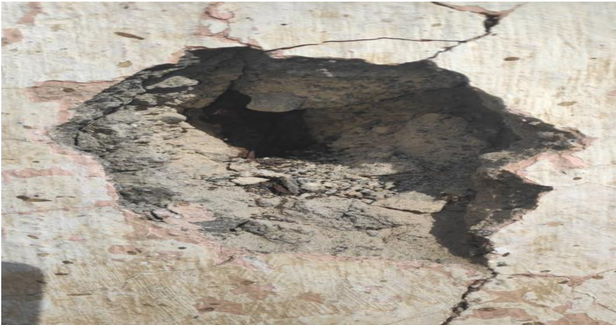
Fig.2– Totally damaged Column
