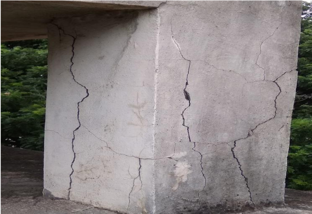
Fig.4– Cracks in water tank column
