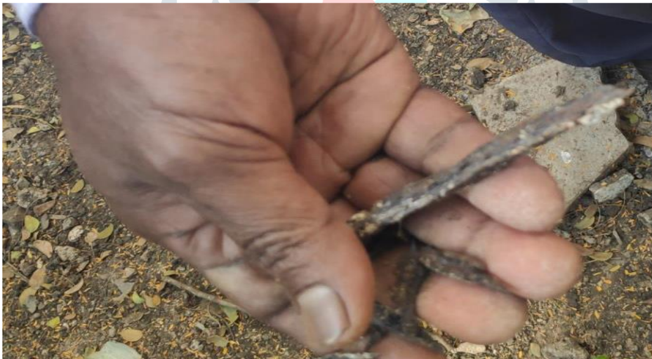
Fig.3– Rusted steel of column
