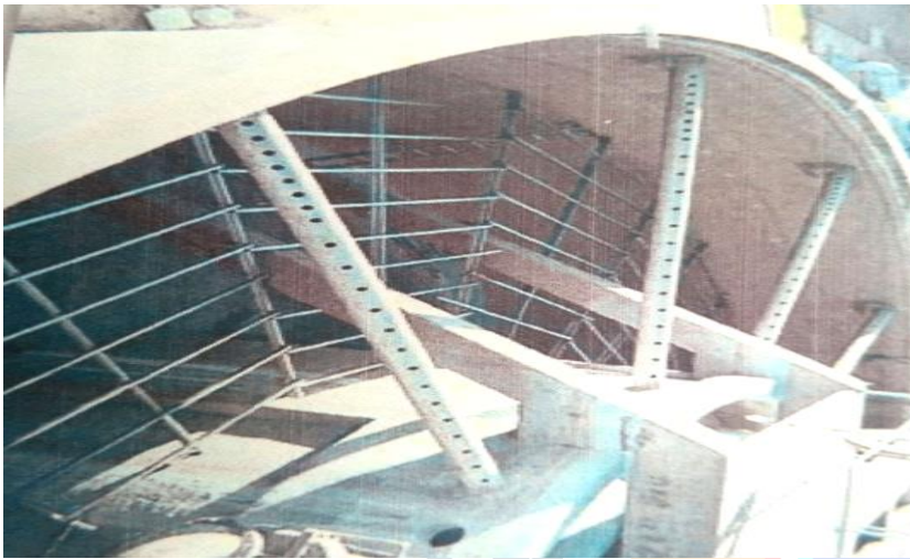
Fig: 4.1a: Tube settler modules placed in Clariflocculator
