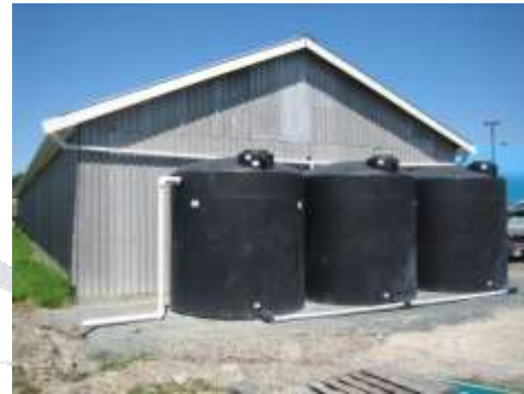
Figure 11: Water harvesting system of a house and connection with water supply channel
