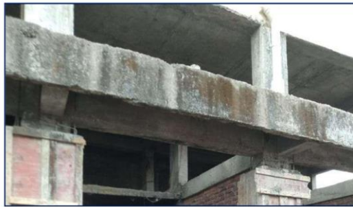
Figure 4.4: Visual Observation of Beams
