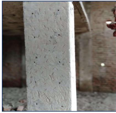
Figure 4.2: Visual Observation of Column
