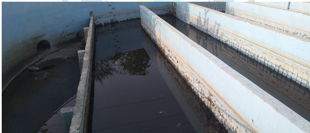
Figure 2 Untreated wastewater at the discharge point of the plant
