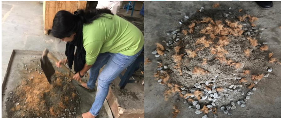
Fig 4.2 Mixing of coir fibre,areca fibre,&amp; plastic waste with cement and other ingredients
