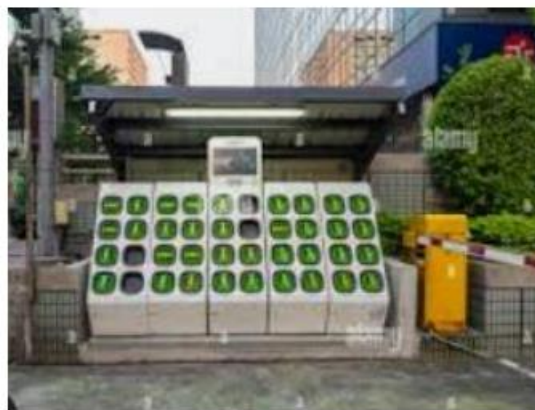
Fig1: batteries at the Gogoro swapping station [10]
