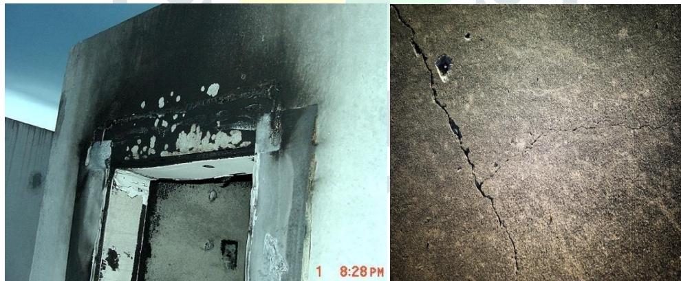
Figure 1.2 Surface of the concrete surface after exposure to elevated temperature
