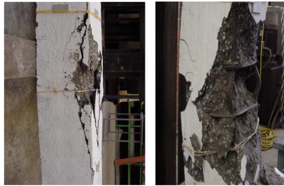
Fig. 4. Failure mode of slender geopolymer concrete columns [15].
