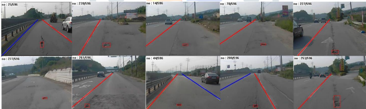
Fig 2. Detected pothole on road
