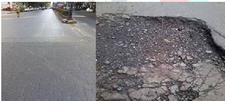
Fig.5 image of plain road and pothole road
