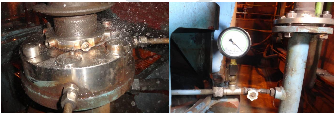
Figure 3 Mechanical seal line vent line having number of connector joint.
