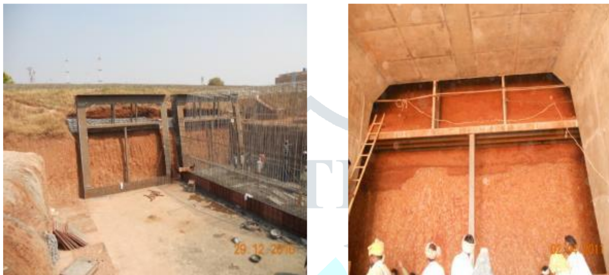
Fig 5: MS Plate/Front Shield for Box Pushing in RUB.
