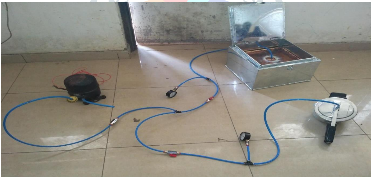
Fig 6: Set – up of the refrigeration system
