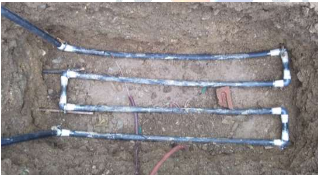
Figure 3.3: Plain pipe used in setup
