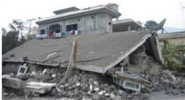
Figure 5 Roof collapse due to a loss of the gravity load-bearing capacity of stone walls in the 2005 Kashmir
