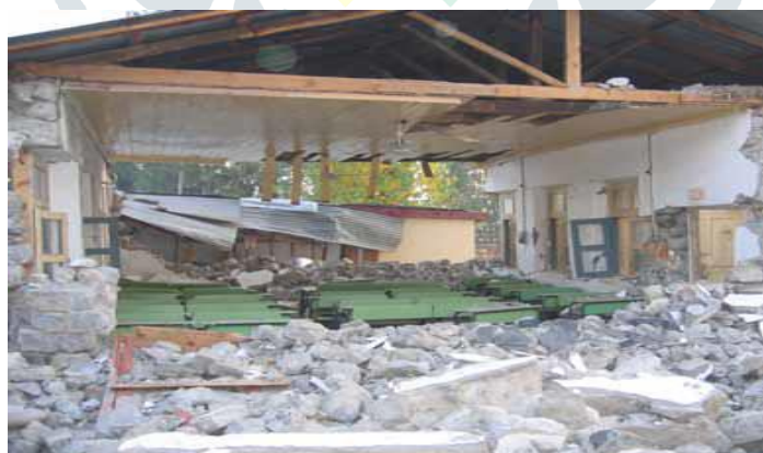
Figure 7 Out-of-Plan Collapses of Two Parallel Walls
