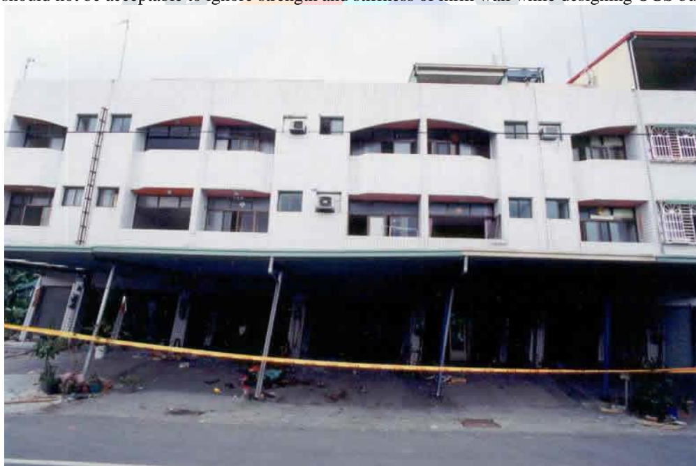
Fig. 1.4: General mode of failure in OGS buildings (Reference: 13)
