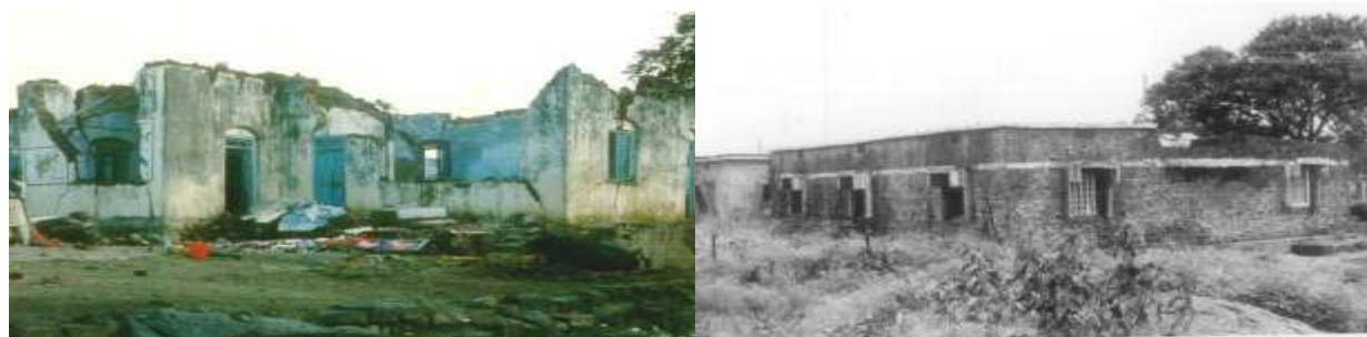
(a) Building with no horizontal lintel band: collapse of roof and walls
