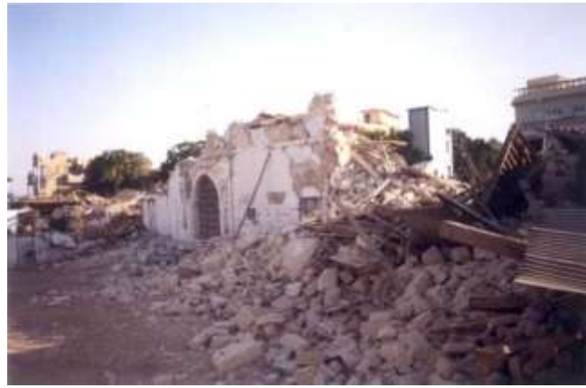
Figure 4: Roof collapse due to a loss of the gravity load-bearing capacity of stone walls in the Rajasthan
