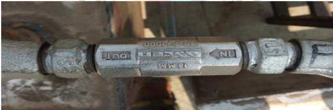
Fig.2.1.5: Flange and NRV
