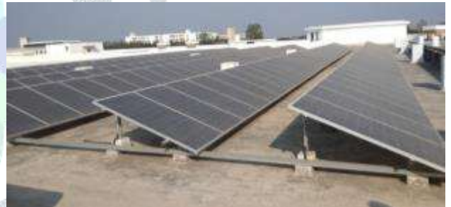
3.1.1) Flat roof mounted solar installation (Sandip Foundation, SIEM, Nashik)
