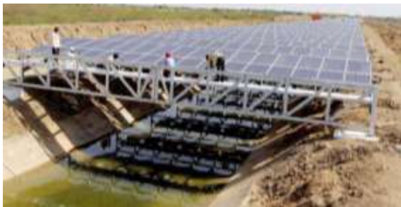
3.15.2) Canal-top PV Solar installation
