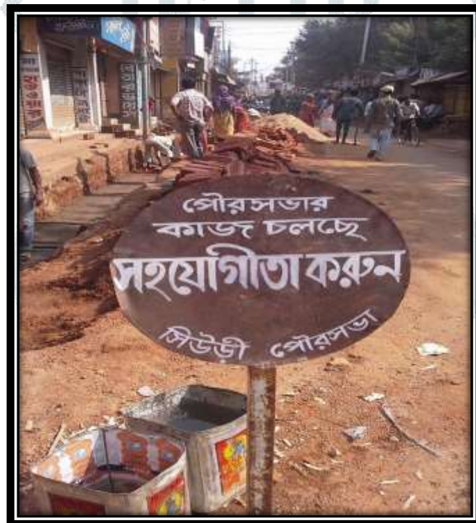
Figure: Constructional work going on at Suri Municipality, Birbhum District, West Bengal
