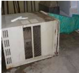
Fig.4 Back side showing air-conditioner and duct
