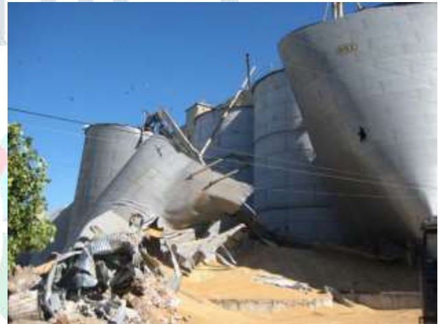
Failure of silo at segment 1 due to excessive Stresses at Junction
