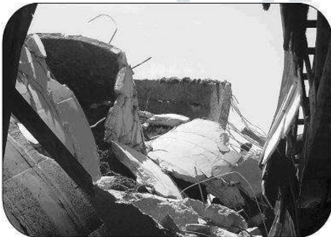
Failure of silo due to earthquake
