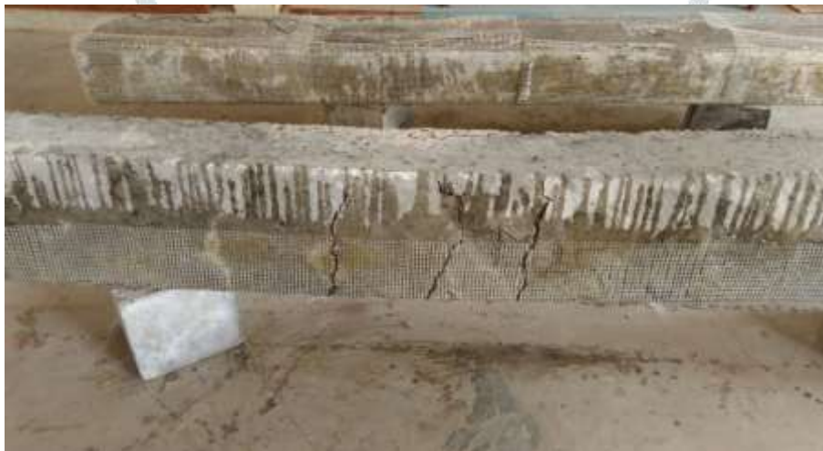
BOTTOM WRAPPED GFRP BEAM FAILURE
