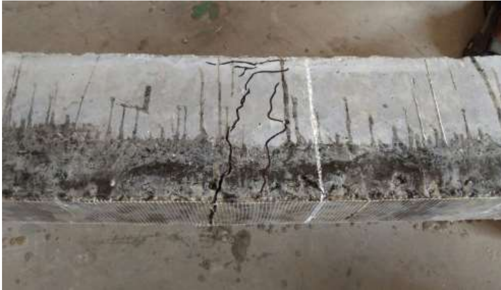
BOTTOM WRAPPED GFRP BEAM FAILURE
