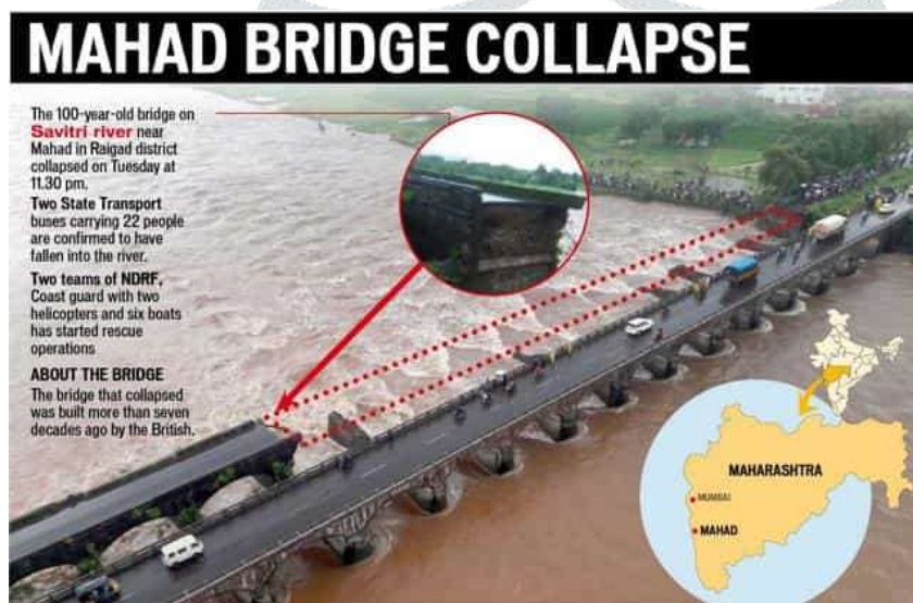
Fig.1. Mahad bridge collapse incidence
