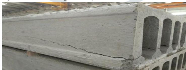
Figure 6.3: Major Crack in Hollow Core Slab
