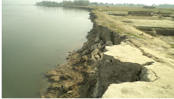
Fig. 2. Eroded river bank at Jiabharali lower plain reach
