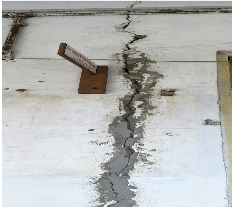
Cracks on the column of SATI building
