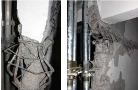
Fig.1.1. Concrete crushing and reinforcement buckling
