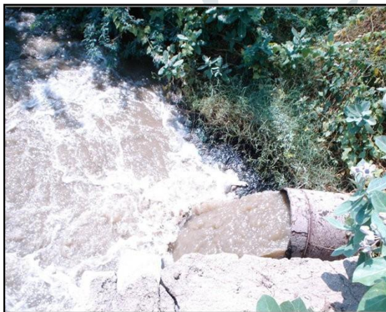
Fig. 6: Treated Sewage Water from the Tirupati Sewage Treatment Plant (STP)
