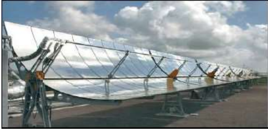
Figure-1: CSP Parabolic Trough Solar Collectors
