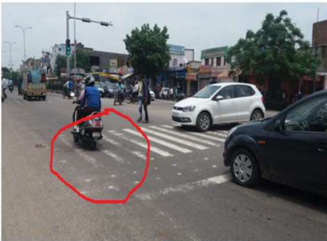
Fig 4 Zebra crossing faded away
