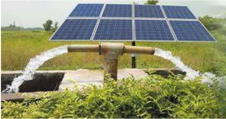
Figure 3- Solar water pump
