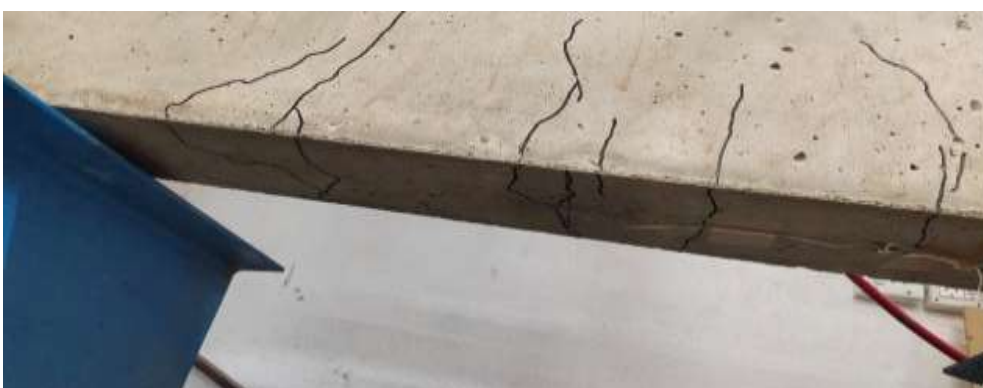
Fig-2: Crack pattern observed form type-1 beam
