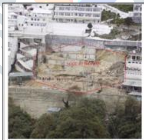
Fig 4. View Of Bhawan Landslide, Katra.
