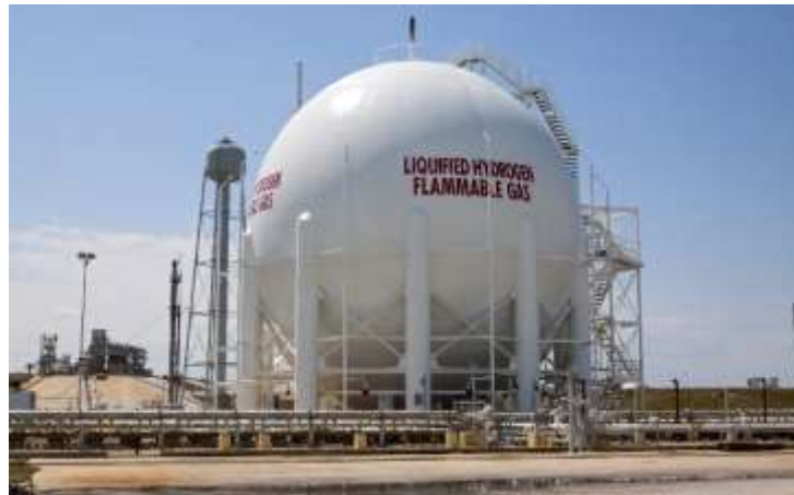
Figure 6 – Liquid Hydrogen Storage
