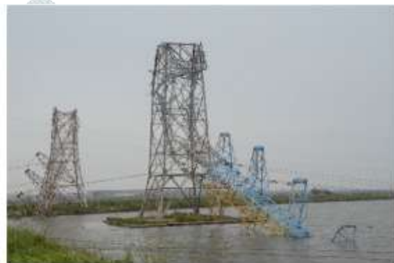
(b) neighboring collapsed tower
