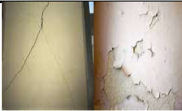
Fig 2: Visual Inspection of Cracks and Damages of Plaster in Building.
