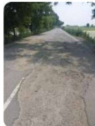
Figure 5 Showing 8m wide road in Bad condition
