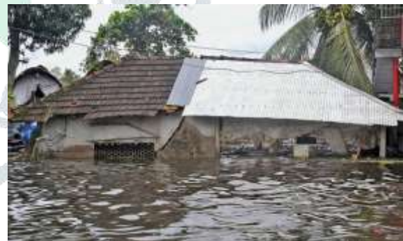
Figure Error! No text of specified style in document. Flood affected house
