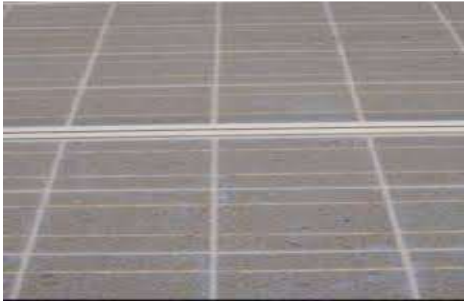
Fig. 3: Solar module covered by heavy layer due to the dust accumulation before cleaning
