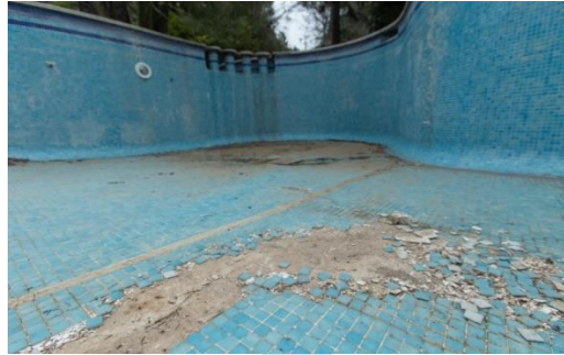
Fig 2 Earthquakes Impact In Pools Flooring
