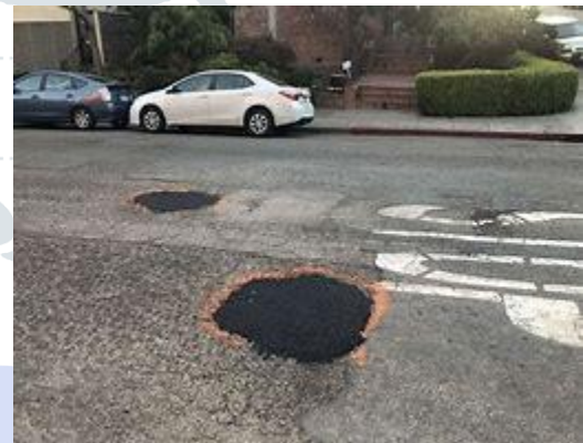
Fig. 1. Condition of roads with potholes.
