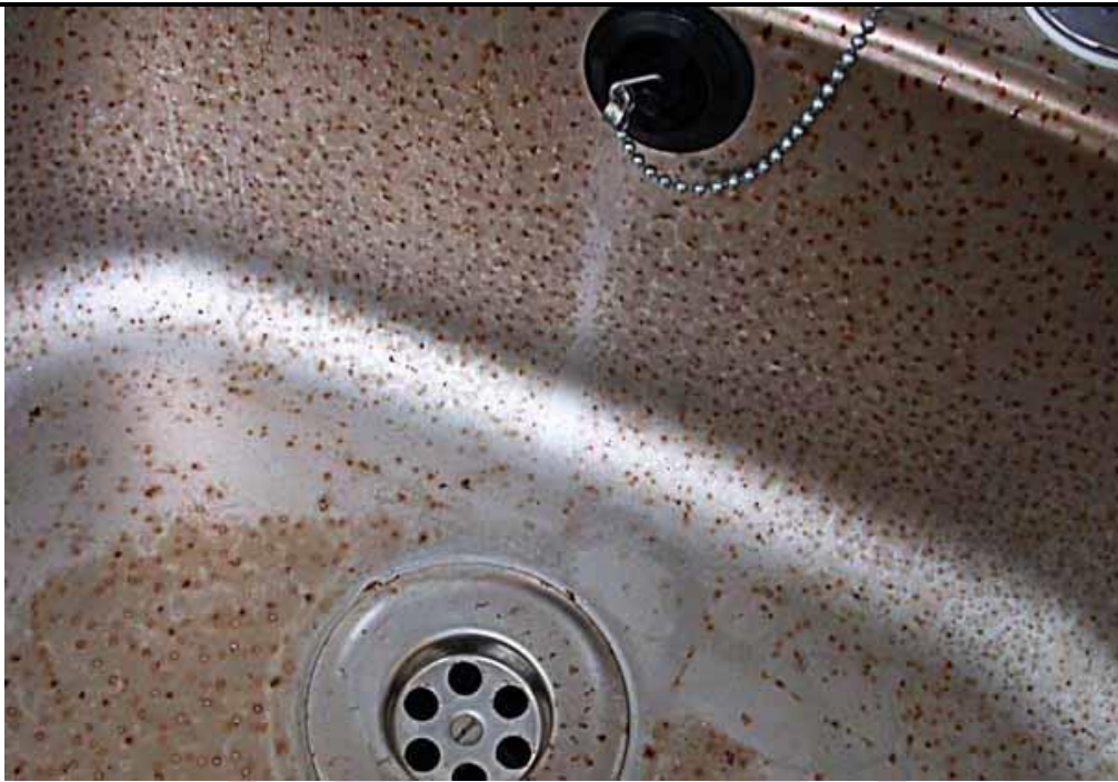
Figure 1.6: Pitting corrosion on sink surface
