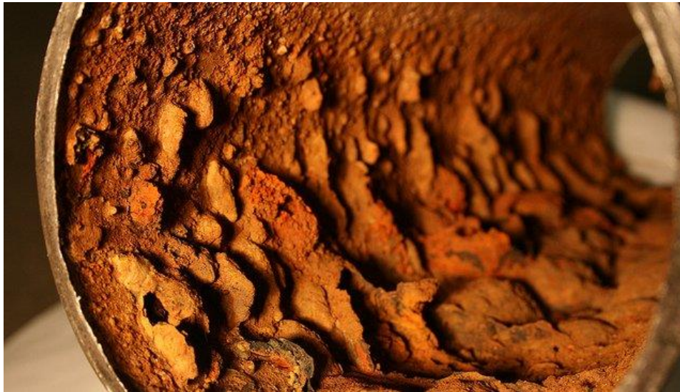
Figure 1.8: MIC corrosion inside a fire sprinkler systems
