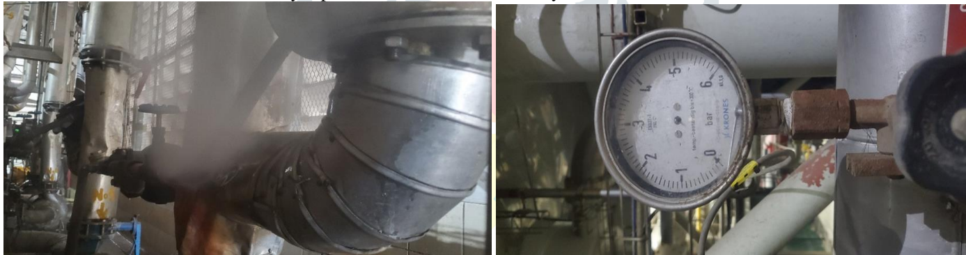
Plate 1: Steam leakage at pasteurizer at packaging and Damaged Pressure gauge with no Pointer ((EABL), 2020)
