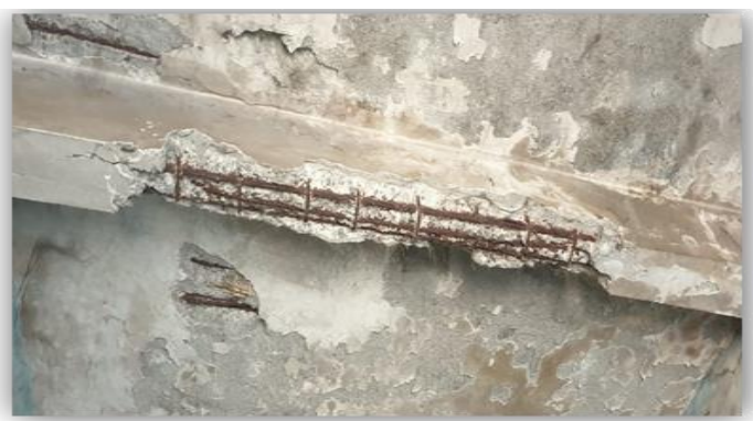
Figure 3.2 Beam steel exposure
