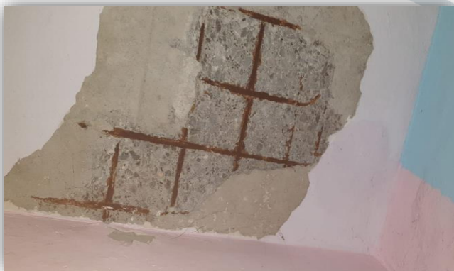
Figure 3.1 Slab reinforcement exposure
