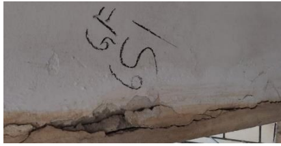
“Figure 5 Cracking due to Poor Construction”
