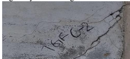
“Figure 4 Cracking due to Shear Stress”
