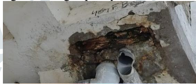
“Figure 1 Cracking due to Structural Overload”
