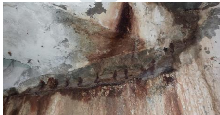
“Figure 3 Cracking due to Moisture”
