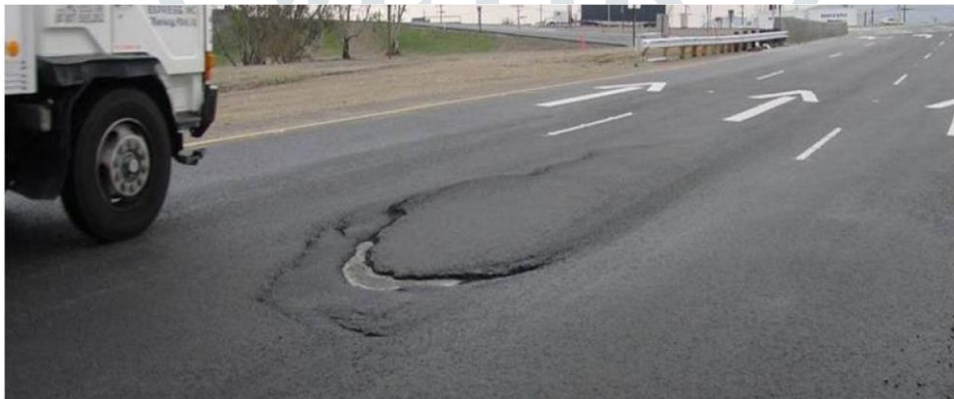
Figure 1.2 Surface Layer Delamination [www.roadscience.net]
