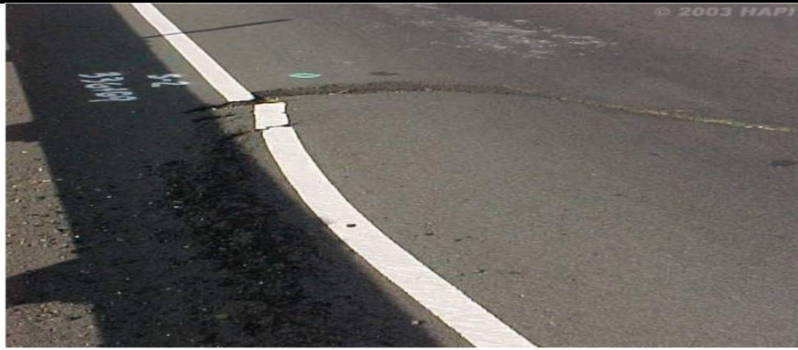
Figure 1.1 Slippage Failure [www.pavementinteractive.org]
