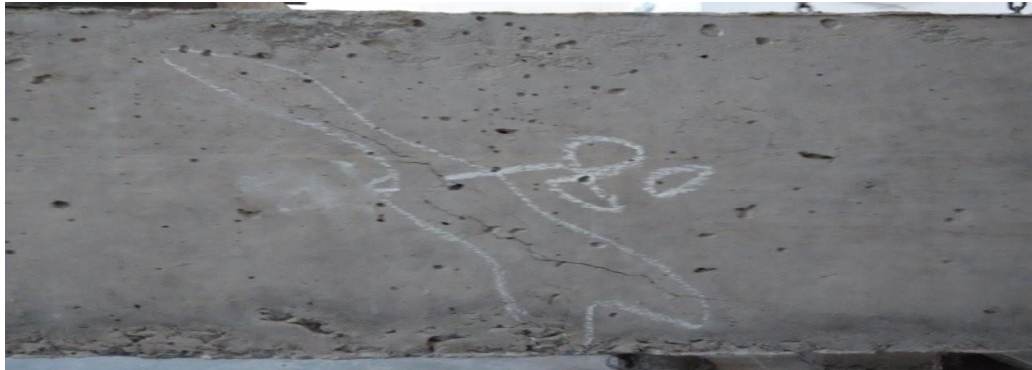
Fig 3.3 First Crack On the Beam
