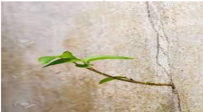
Fig.6 Fracturing Due to Vegetation
