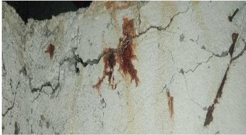
Fig. 2 Fracturing due to thermal stress
