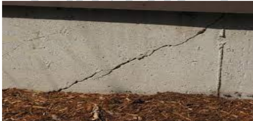
Fig. 1 Fractures due to Moisture
