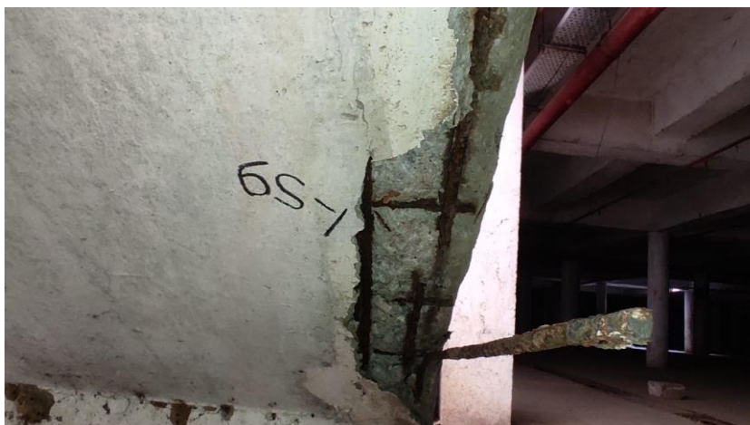
Fig 4. Fracturing due to swelling of reinforcement
