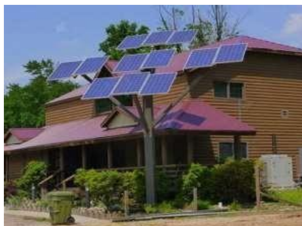
Figure 5 Mounting of Solar Tree near the house
